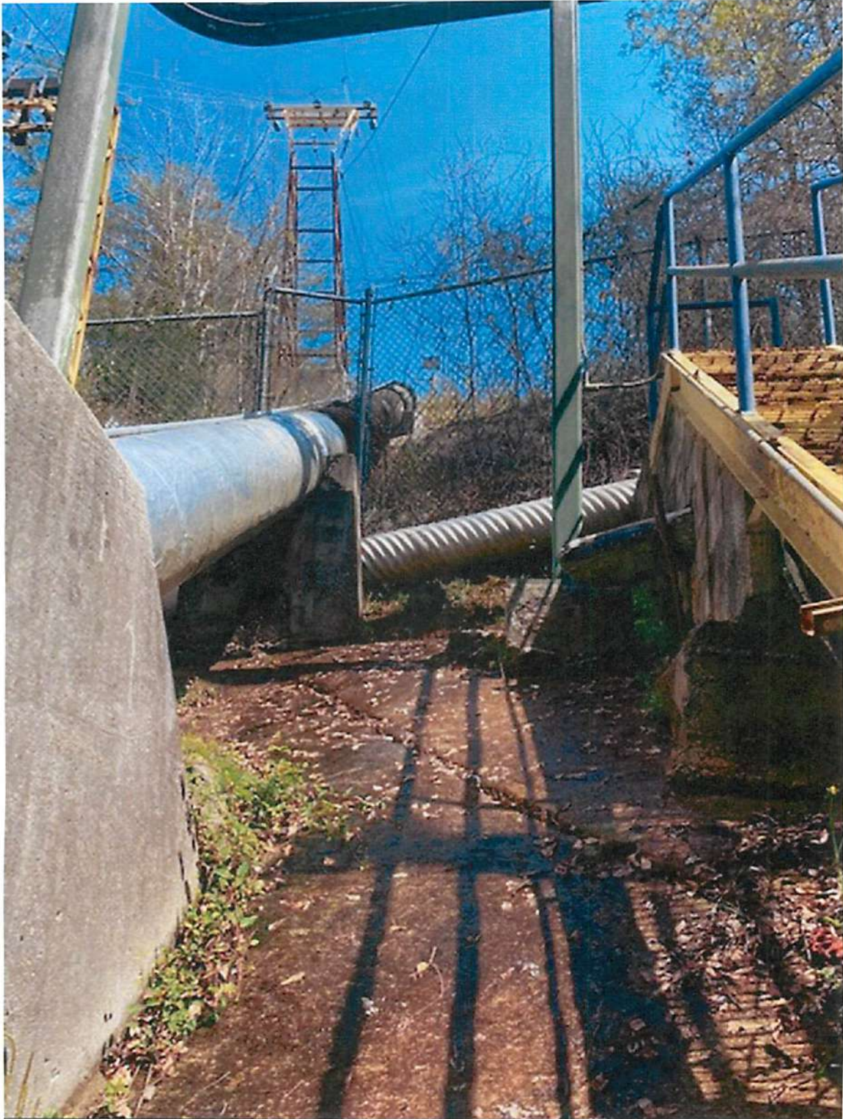
View from the bottom of the hill looking up to the top of the hill where the check valve building is located. This is a 24" water line from the river intake to the water treatment plant 2 miles away. The cost of wiring from the bottom of the hill to the top of the hill is $105,000.00
