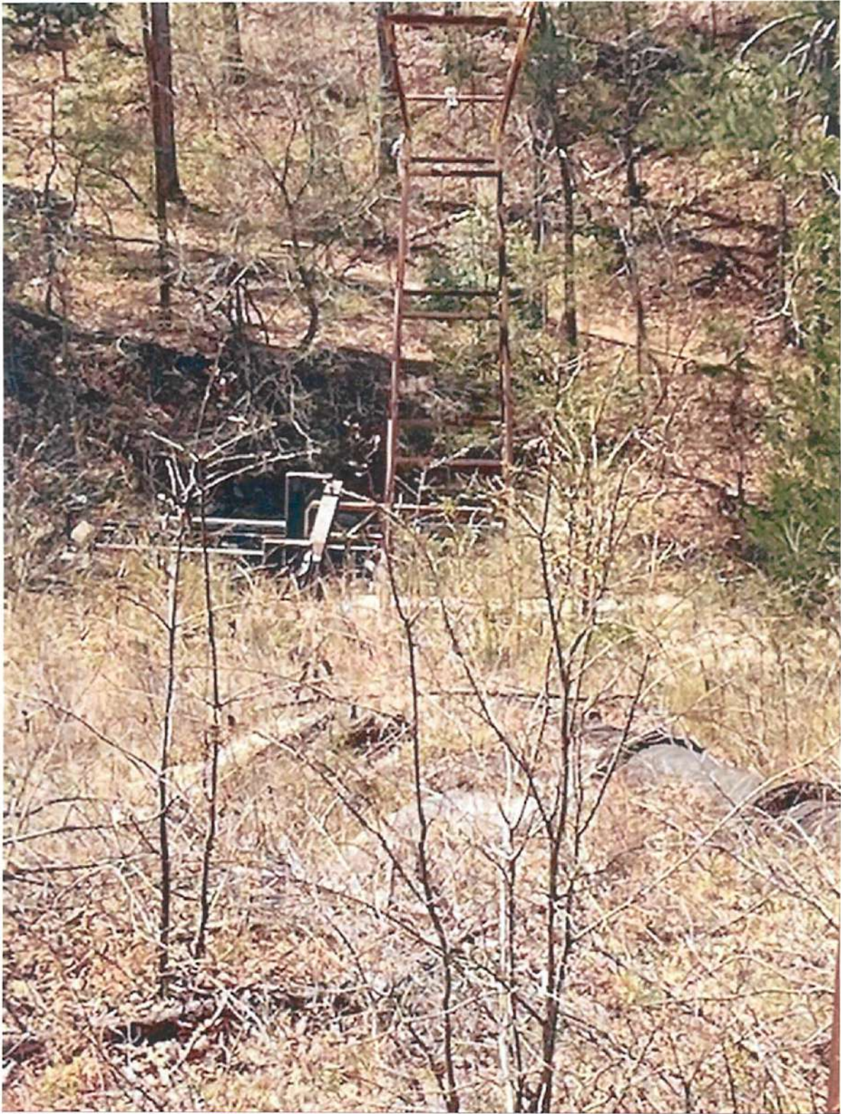
This is a view from the top of the hill where the check valve building is located down to the mezzanine where the pumps & motors are located. The 24" water line is partially underground.
